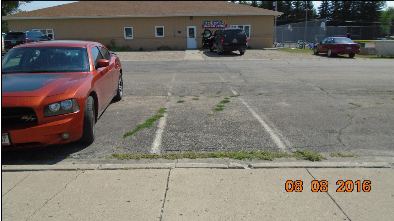
Figure 6. Ramp missing at the crosswalk connecting the park and the daycare center
