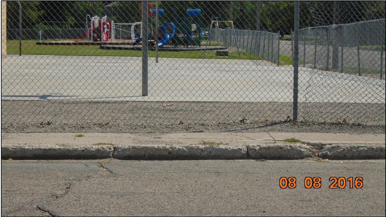
Figure 12. Gravel on sidewalk at the west side of elementary school
