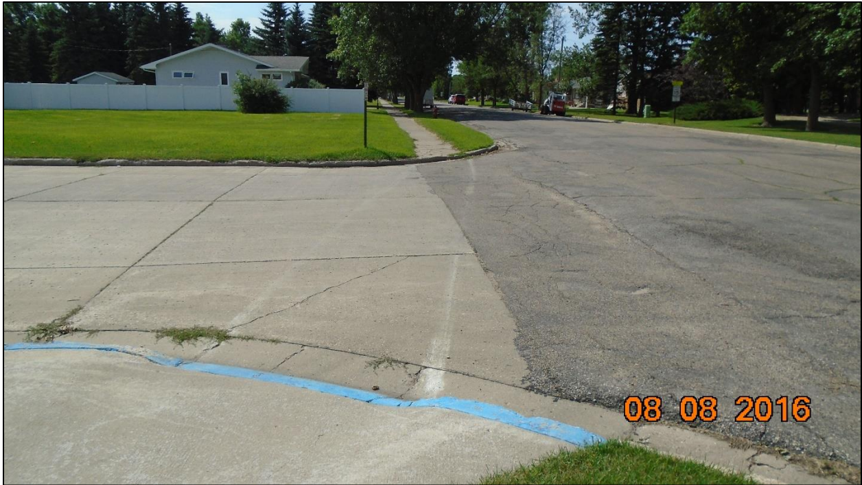
Figure 4. Ramp missing at the end of crosswalk at southwest corner of high school
