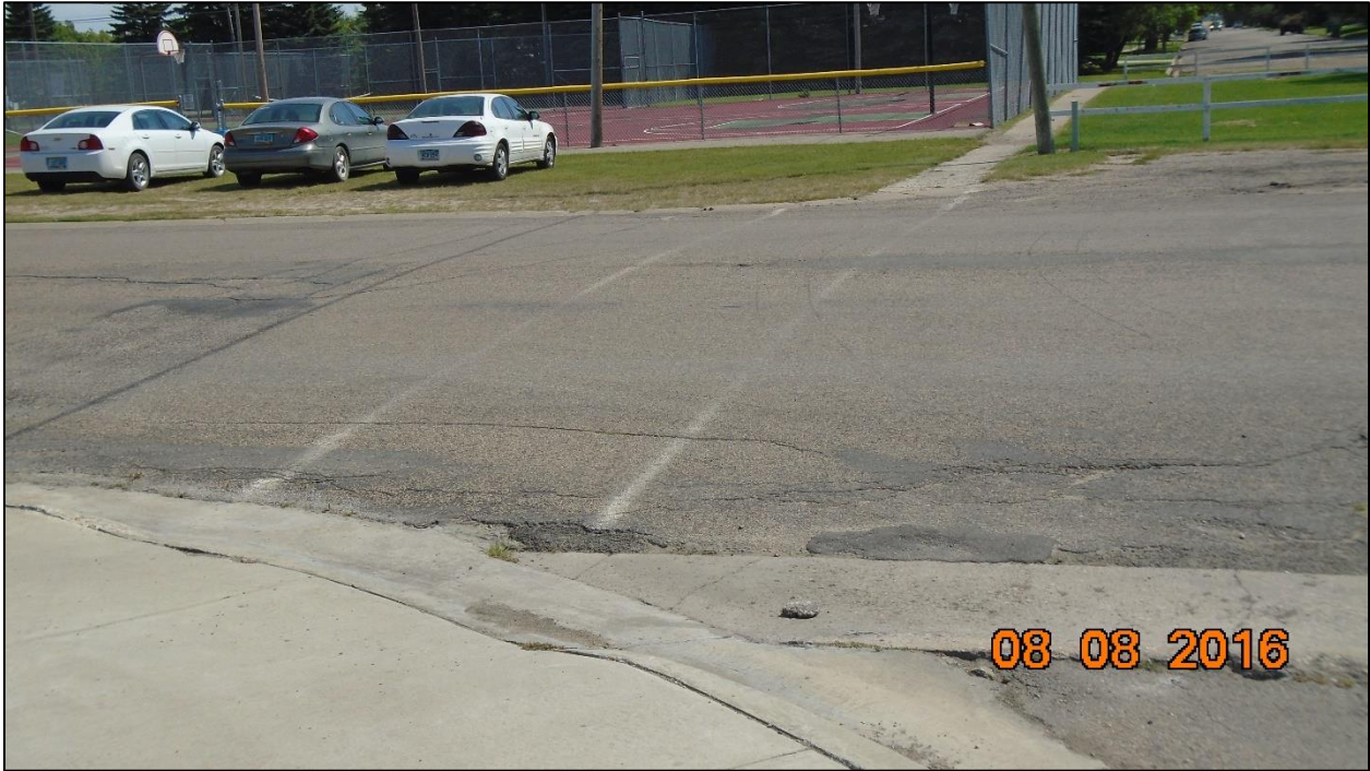
Figure 10. Faded pavement marking at northeast corner of elementary school
