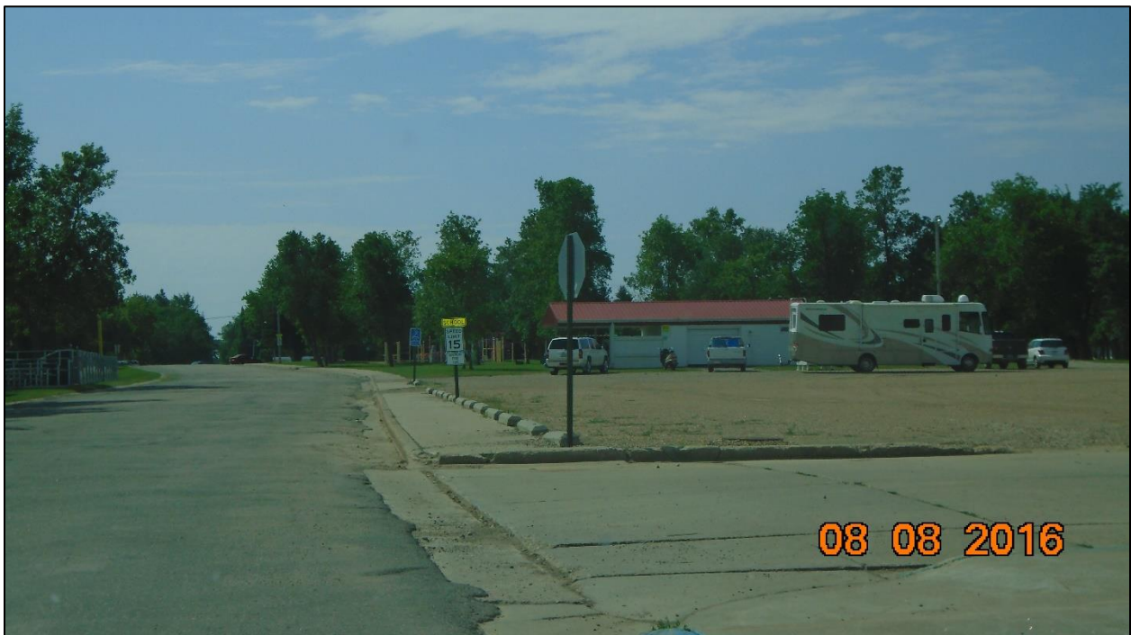
Figure 5. Ramp missing at the end of crosswalk at southeast corner of high school
