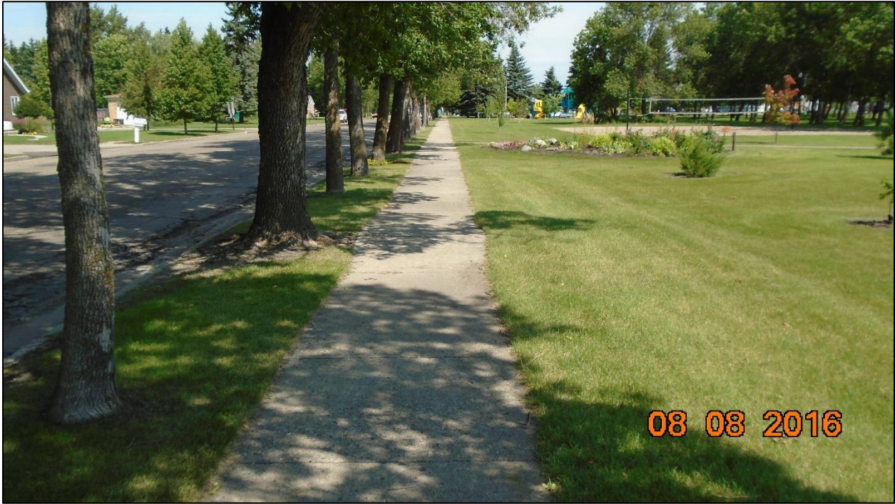
Figure 13. Heaved sections of sidewalk on the west side of park.
