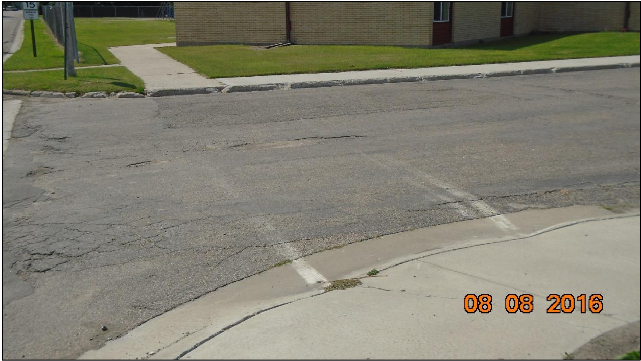
Figure 11. Another faded pavement marking at northeast corner of elementary school
