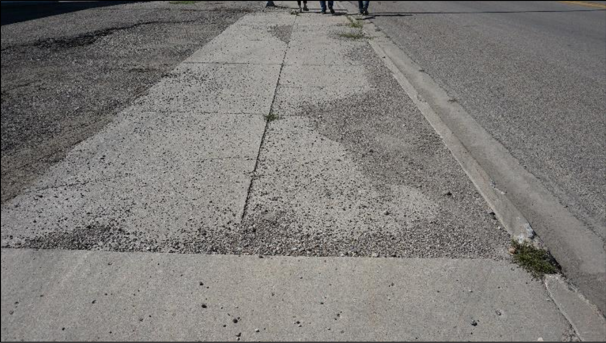
Figure 19. Debris and weeds on the sidewalk
