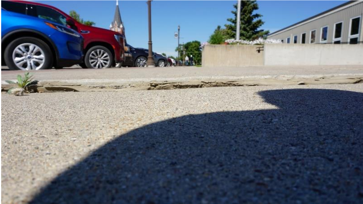
Figure 20. Sidewalk displacement along Third Street
