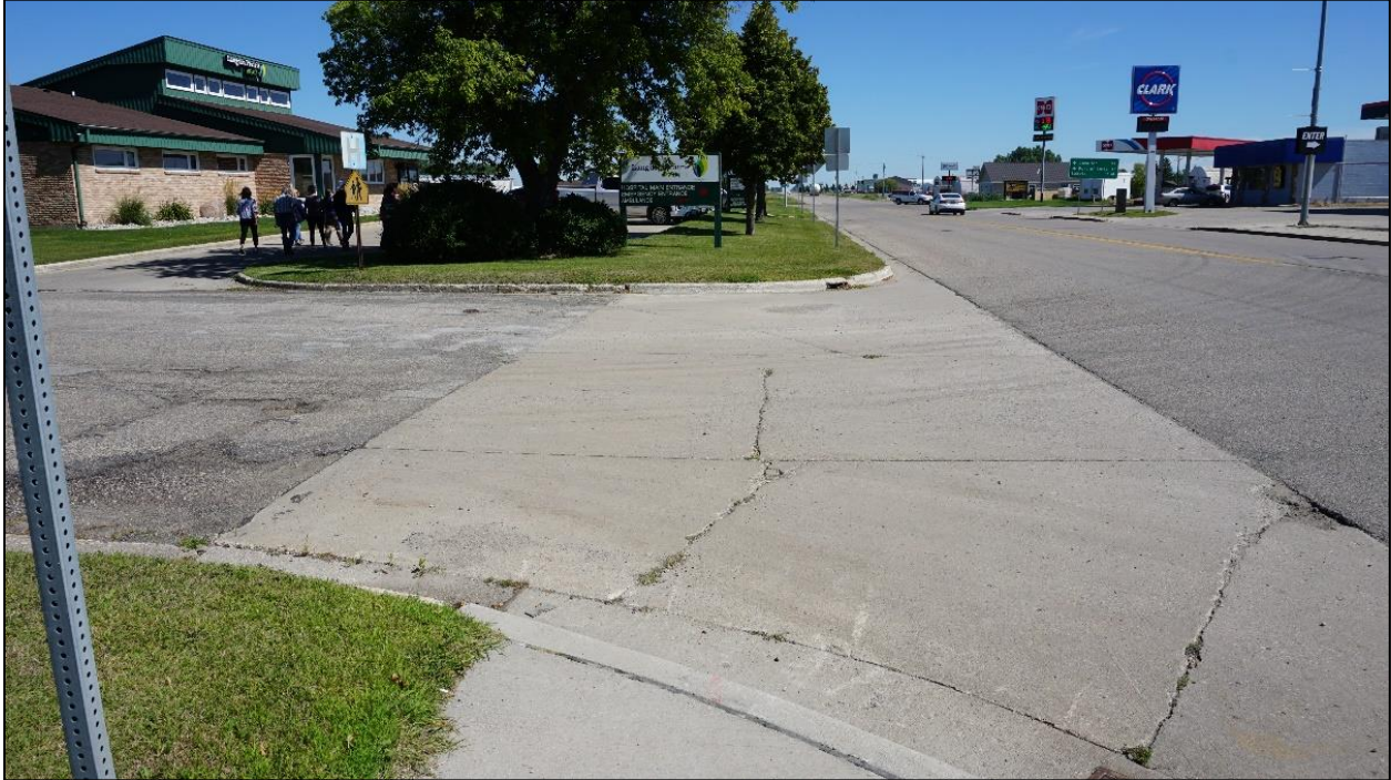
Figure 5. Missing ramps, crosswalk and sidewalk along ND Highway 5 and participants walking through parking lot
