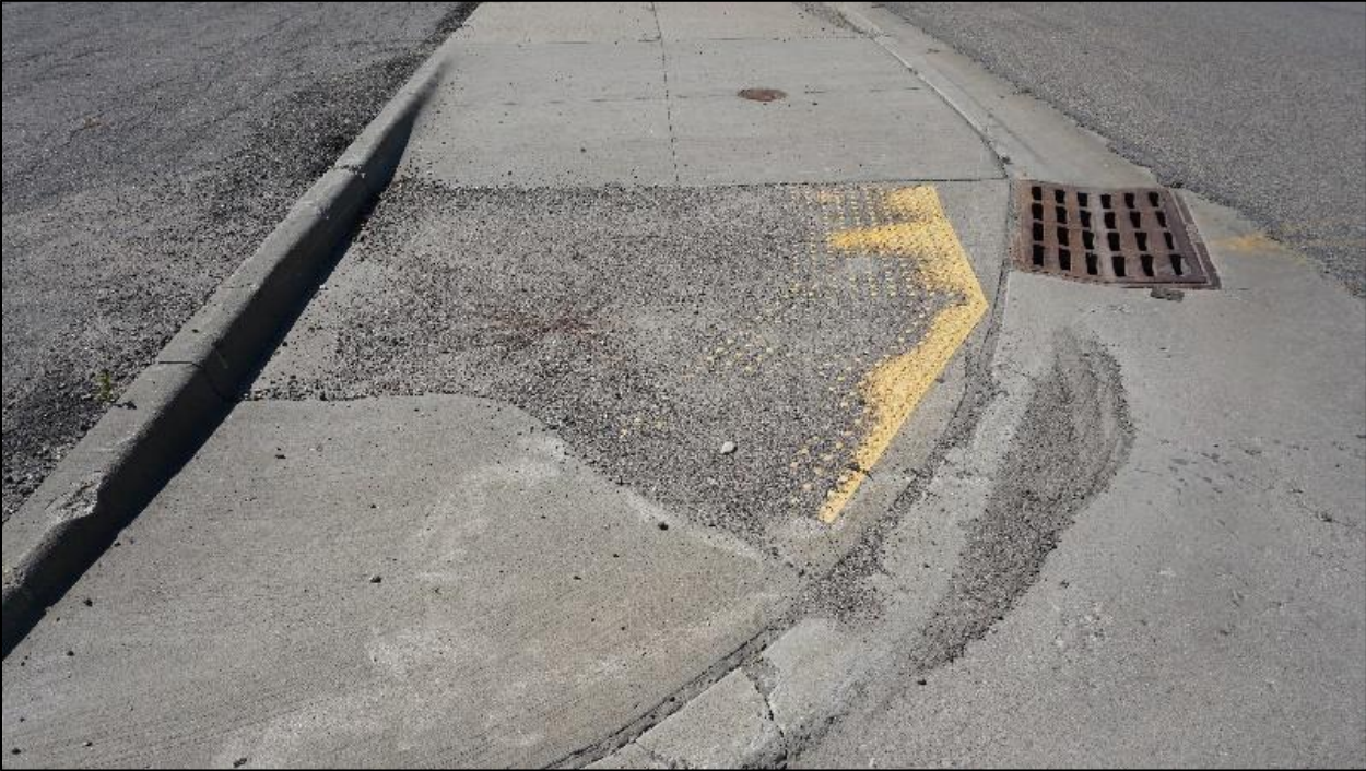
Figure 18. Debris strewn across ramp and potentially hazardous grate
