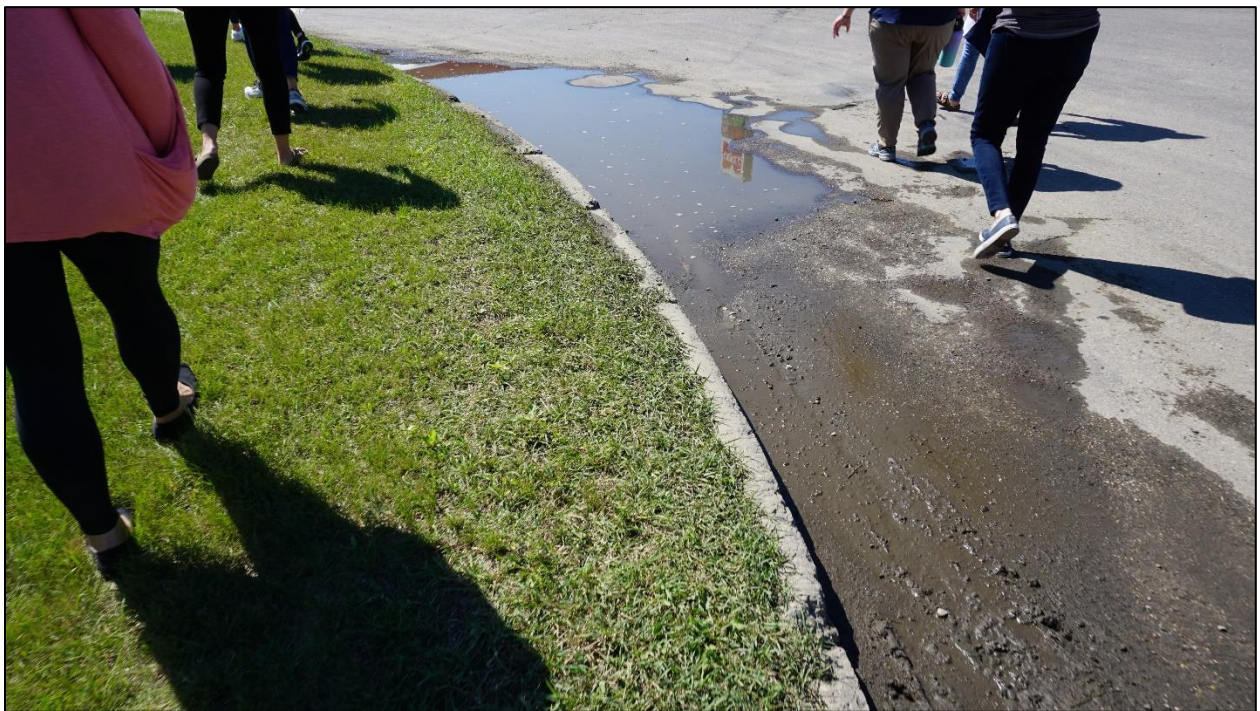
Figure 13. Puddled water at the southeast quadrant of the intersection of ND Highway 1 & ND Highway 5
